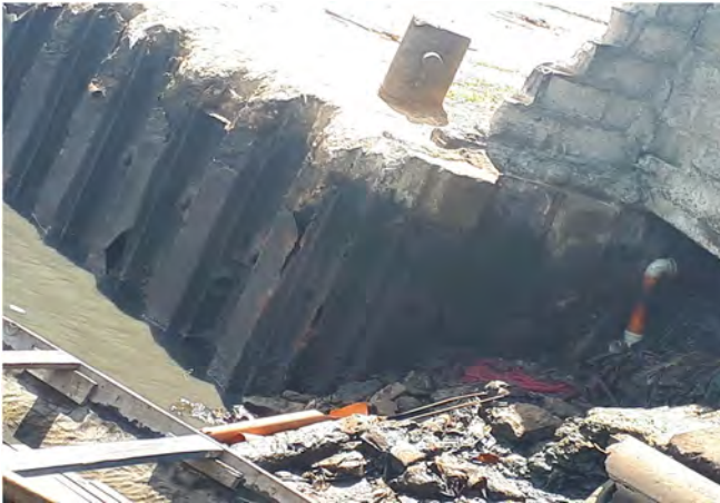
Figure 15: Sewage piped directly into creek water, near Abuloma Jetty
