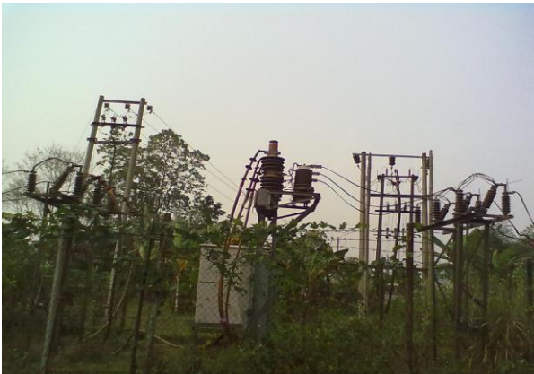
Fig. 6: Power plant with ceramic insulators
